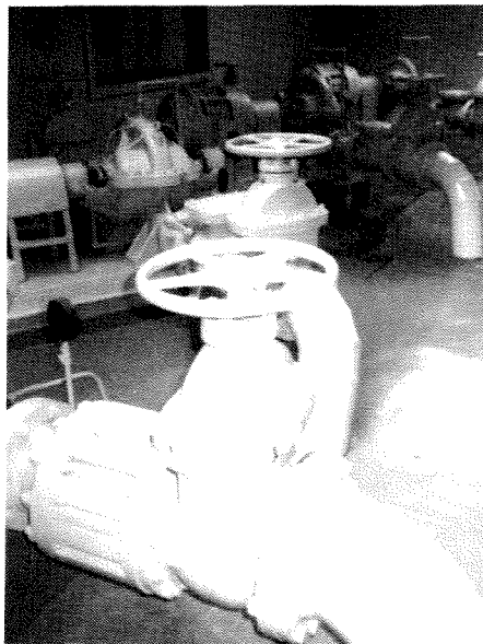
Pumps still functioning in the pumping station at the Old Water Yard on Elm Street.
